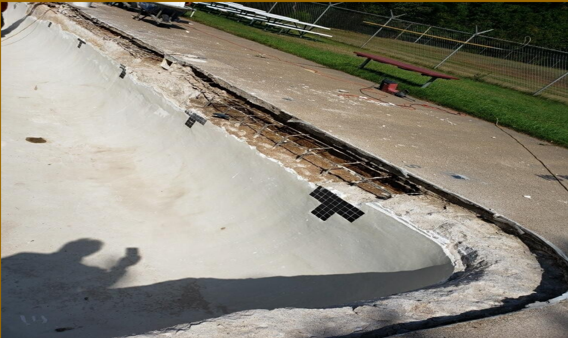
Olde Mill Pool with new tiles and plastered walls, coping Tiles and painted lane markers.
